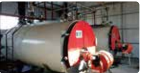
Boiler Heating 锅炉加热
